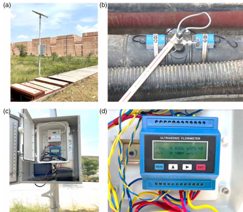
Figure 5 | Hydraulic Node 27 and its components. (a) Above the ground unit with solar panel. (b) Ultrasonic flow and pressure sensor mounted on supply pipeline control panel. (c) IP67 enclosure for housing IoT devices. (d) Flow meter display screen.
